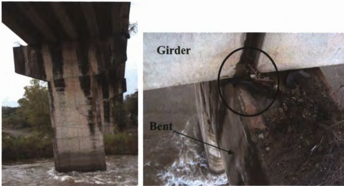
Figure 5-10: Bridge Pier Tilted and Rotated During Earthquake
