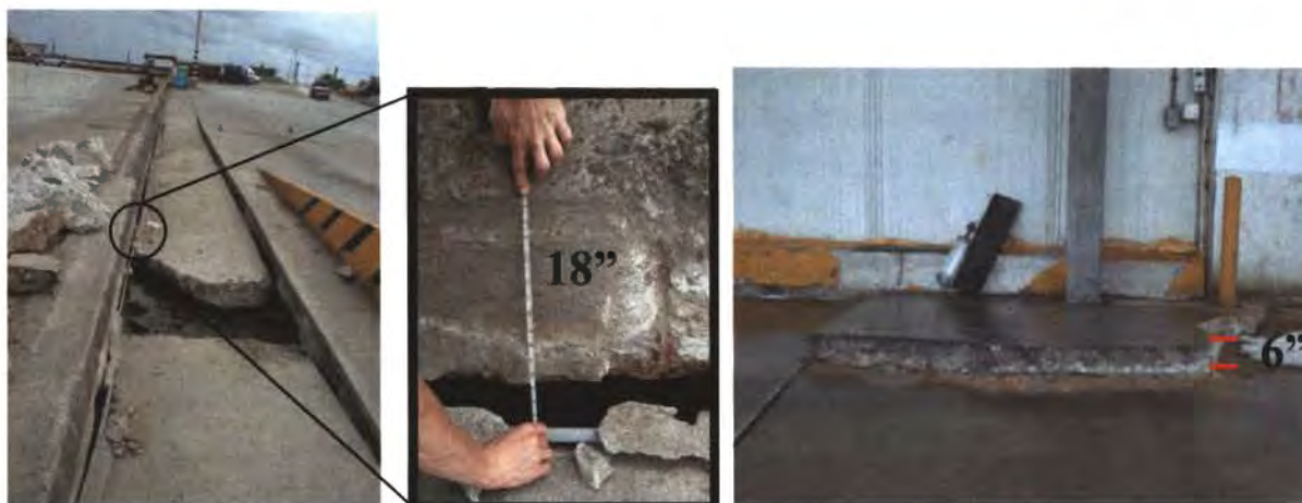
Figure 5-7: Subsidence and Differential Settlement at Puerto Cortes
